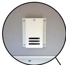
Ventilation system with thermo-fuse
