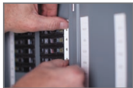
Breakers and Modules
