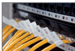
Cables and Wires
