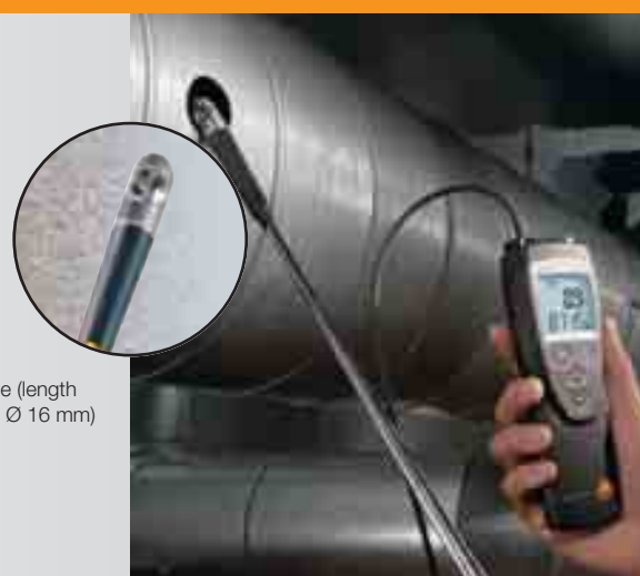
Monitoring air velocity in air conditioning ducts
